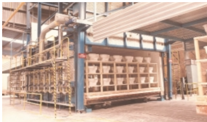
A typical traditional kiln furniture arrangement for a sanitaryware shuttle kiln.
