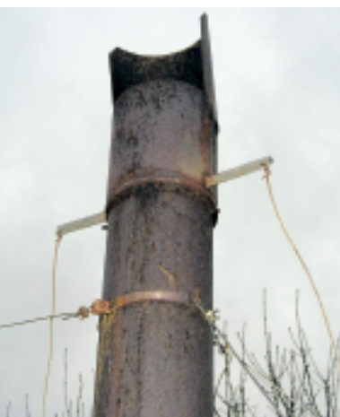
Top: The new enclosure for Kiln #2. Above: Chimney cowl with adjustable top.
